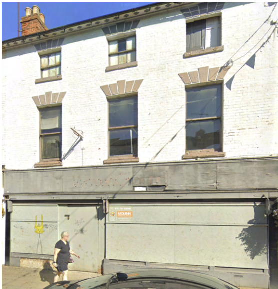
Previously boarded up for several years
